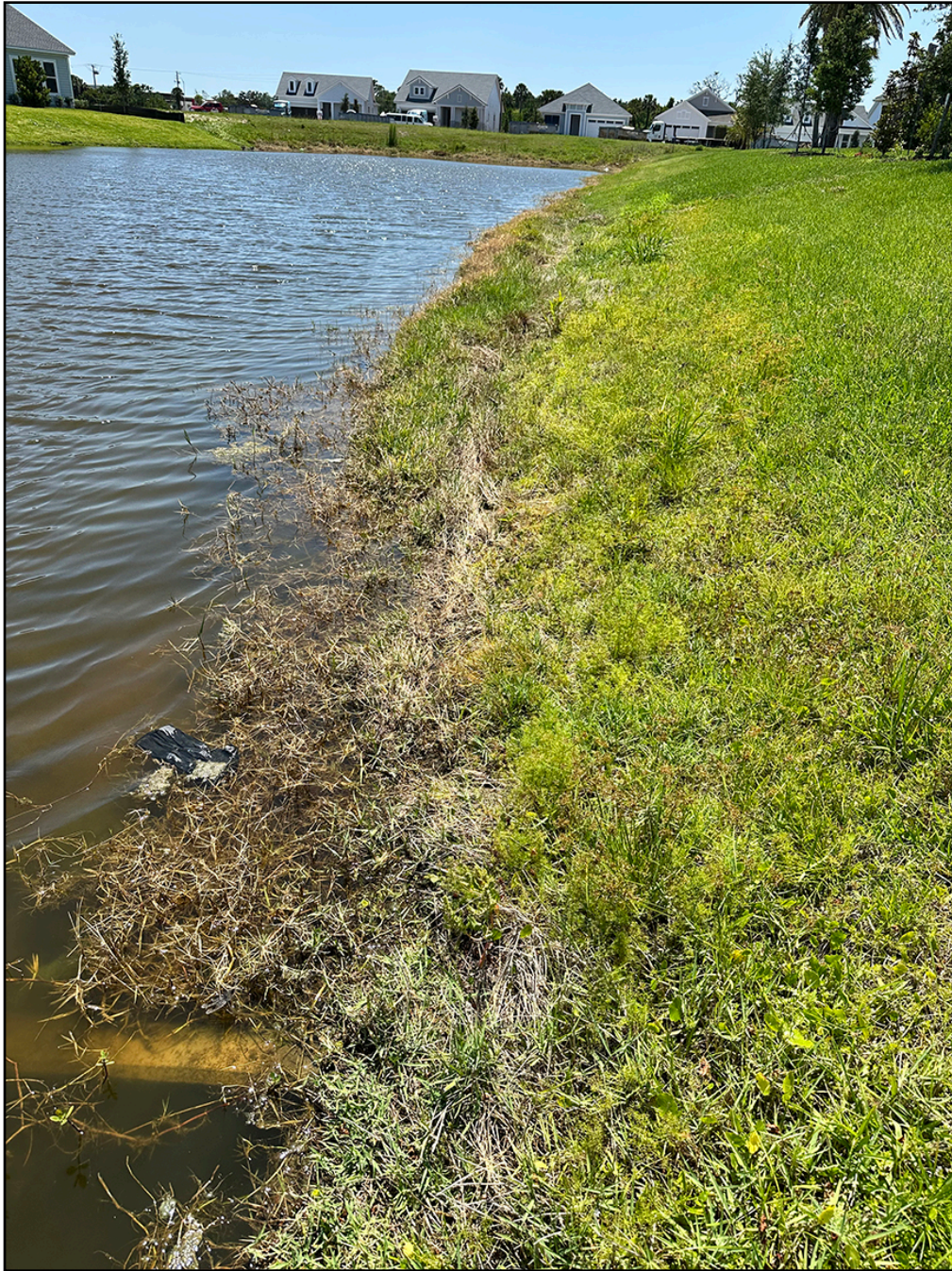
Figure No. 7- Pond #11 undetermined end of bank due to lack of proper vegetation maintenance.
