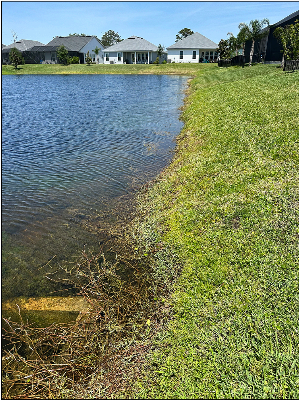
Figure No. 5.- Pond #9 bank separation from the submerged invert.
