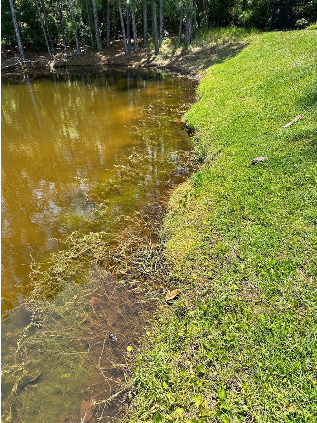
Figure No. 3 - Pond #6 irregular shoreline due to loss of bank sediment.
