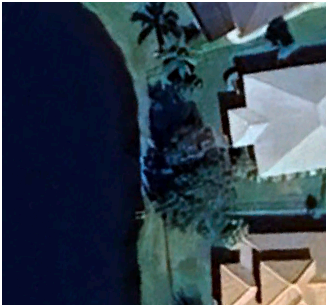
Figure No. 4 - Pond Bank - 87 Pintoresco October 2024- bank has eroded approx. 2' exposing invert.
