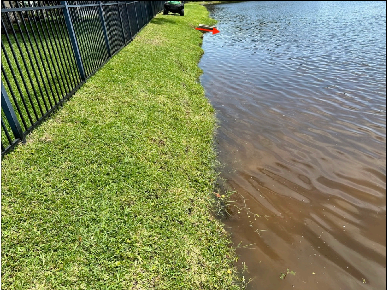
Figure No. 7.- Current pond bank condition between fence line and waters edge 87 Pintoresco Dr. Showing loss of embankment exceeding 2.5' North of the street invert.
