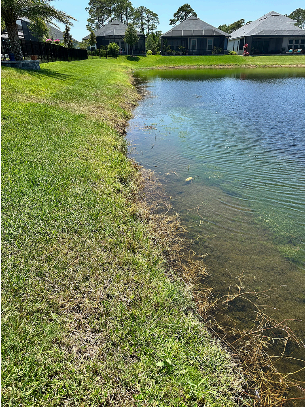
Figure No. 4 - Pond #9 shoreline erosion exhibited by irregular bank topography.
