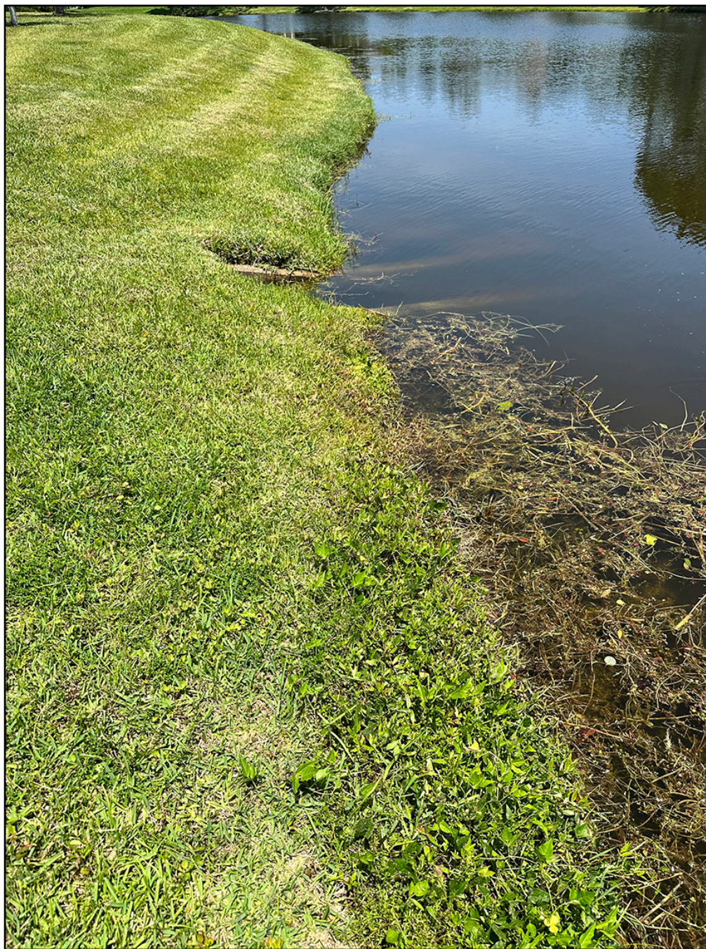
Figure No. 2: Pond #6 Lake bank area exhibiting slope issues cause by erosion.
