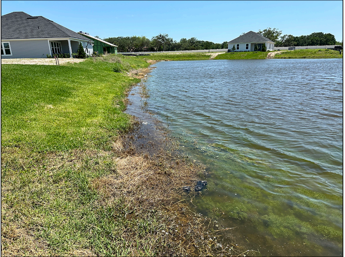
Figure No. 6.- Pond #11 various levels of erosion effects along the entire embankment.
